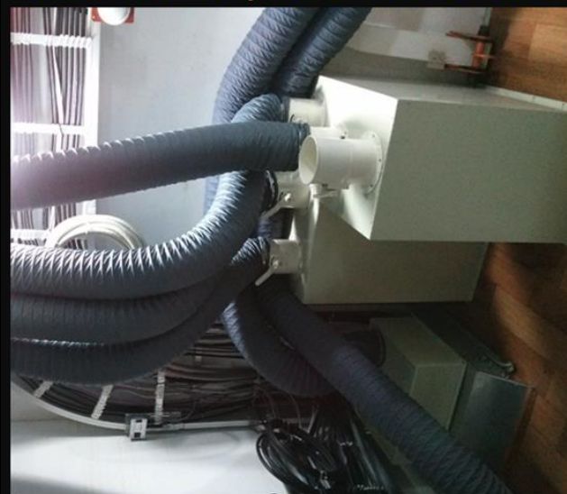
New thermal control system at KVN Yonsei Rx Room
