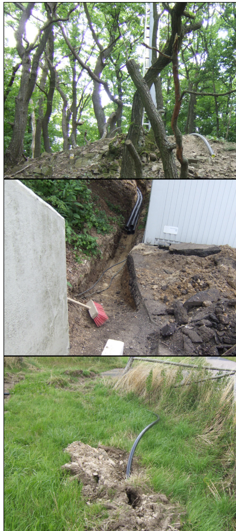
Figures: Pictures from the Effelsberg fiber installation provided by Faron, the company executing the work.
